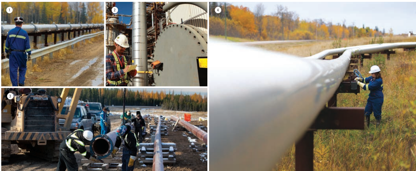
1. Inspection of piping at Cold Lake Operation. 2. Testing of pressurized equipment before the startup of Kearl Oil Sands. 3. Pipeline preparation for the Nabiye project. 4. Wildlife cameras in use at Cold Lake.
