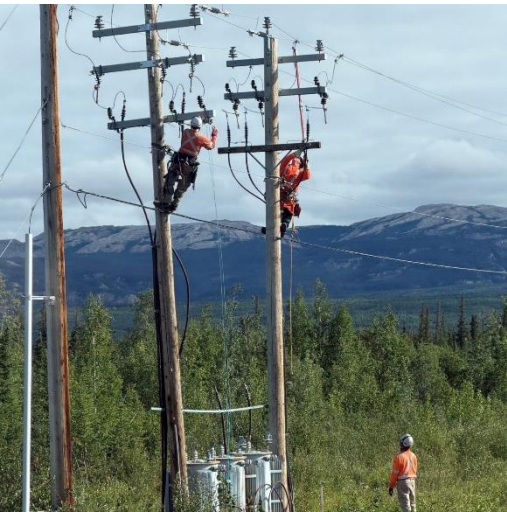
Energy transition to Northwest Territories Power Company
