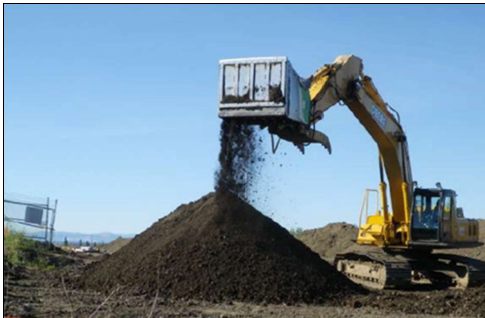
Image H: Biocell Treatment – Aeration/Twister Bucket
