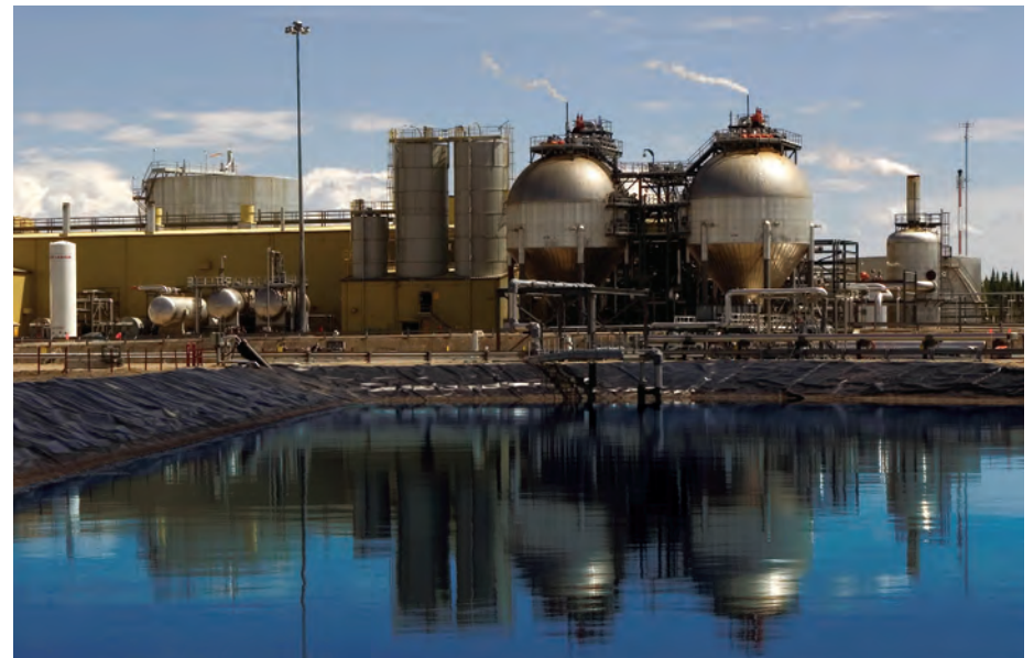
Top: Muskeg Lake near Imperial's Kearl oil sands development was built to replace fish habitat that was disturbed by development. Bottom: Water management infrastructure at our Cold Lake operations.
