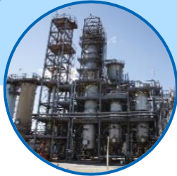
First lube oil hydrofining
